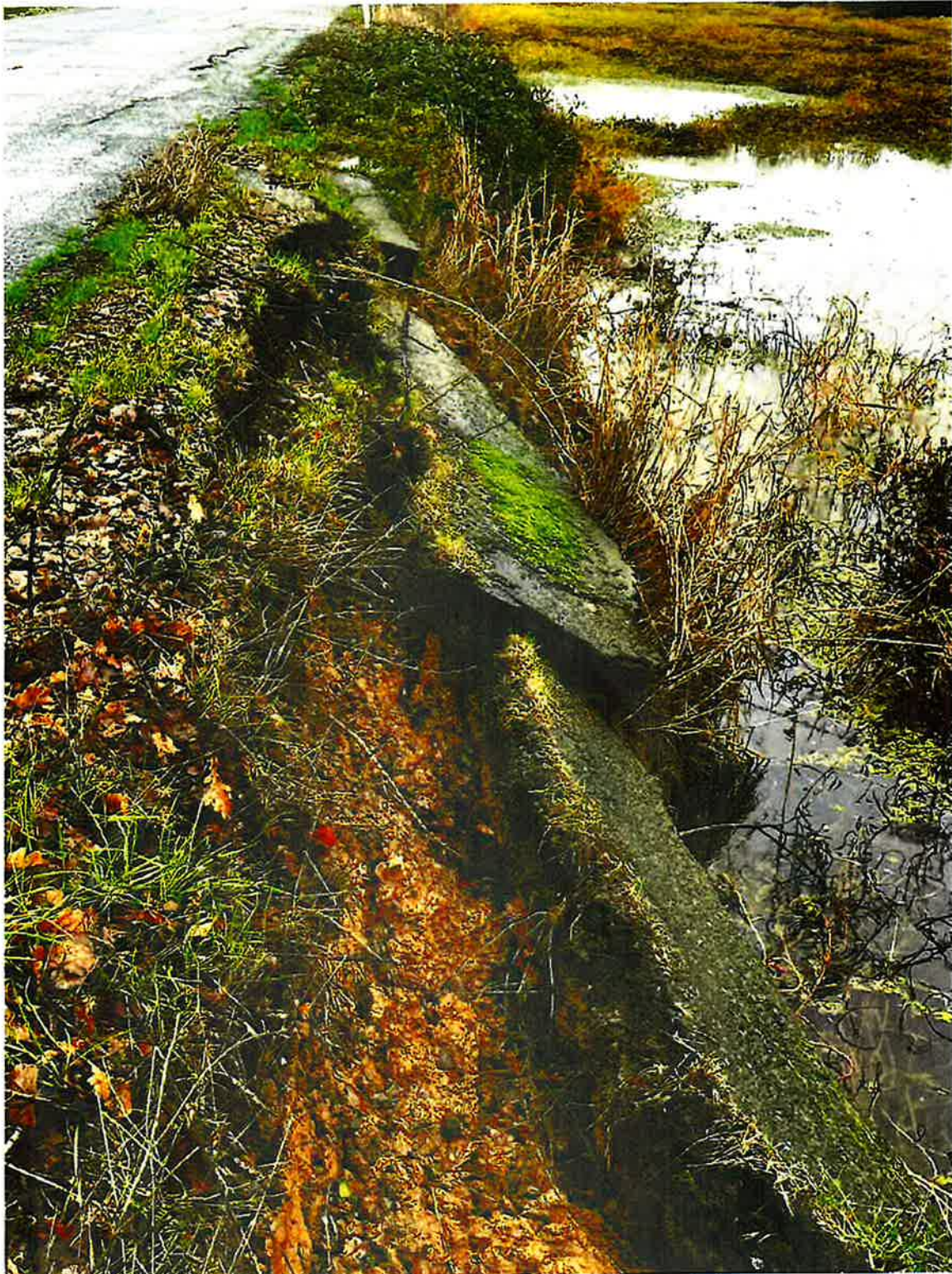
PHOTO 4: PREVIOUSLY REPAIRED SITE PRE-REPAIR CONDITION
