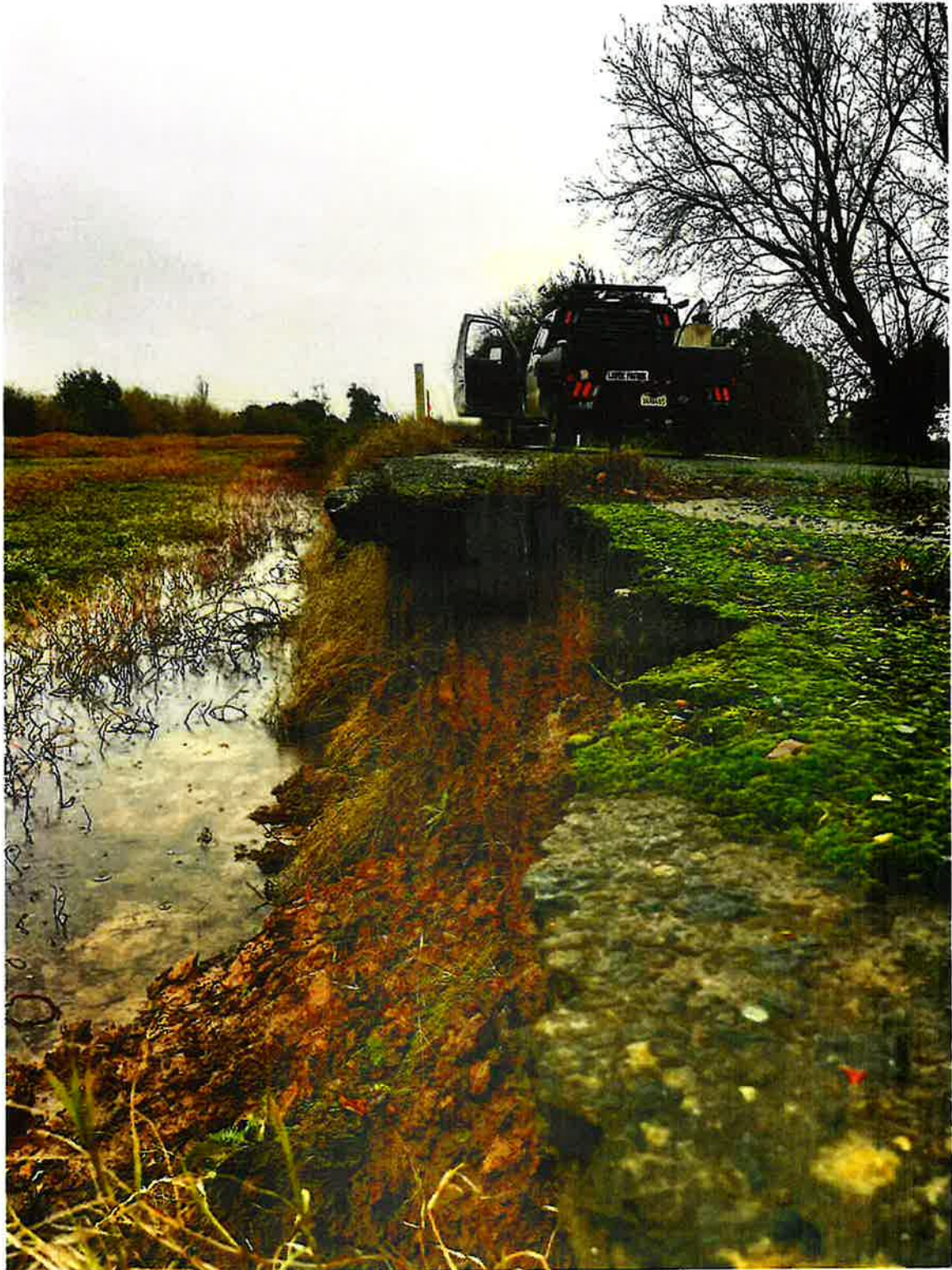
PHOTO 3: PREVIOUSLY REPAIRED SITE PRE-REPAIR CONDITION
